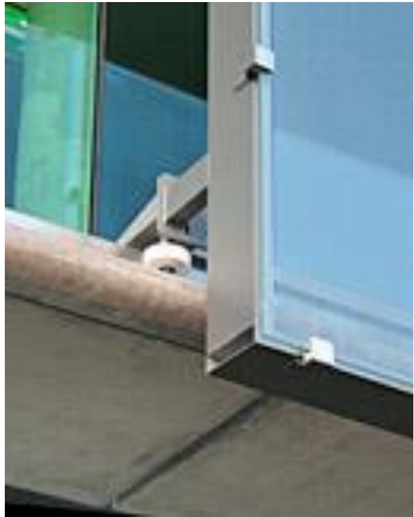
Figure 1-12: Details of photovoltaic panel (Web A-08)
